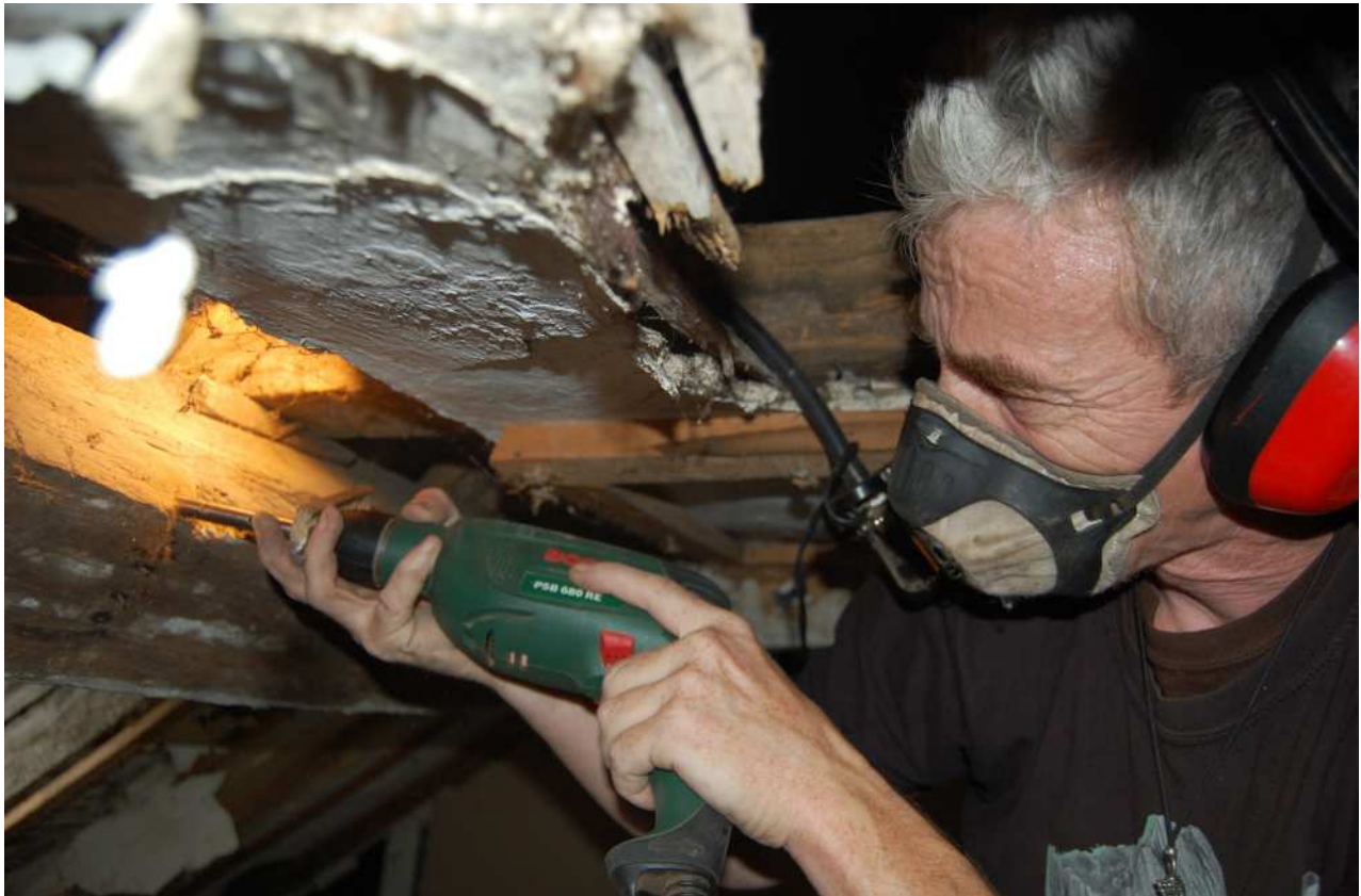
Taking a small core from roof timbers using a 12mm hollow auger
